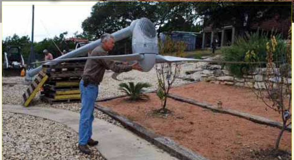
Kevin Christiansen of RePower Engery checks out the blades of a wind turbine he prepares for installation at a Kerrville home where the owner was looking for independence from utility companies.
